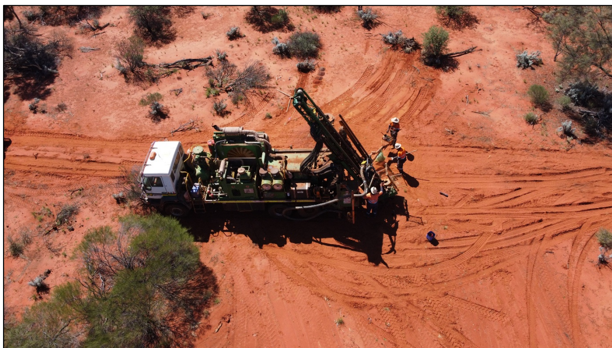
Figure 1. Image of the Air-core Drill Rig operating as part of the current drill program.
